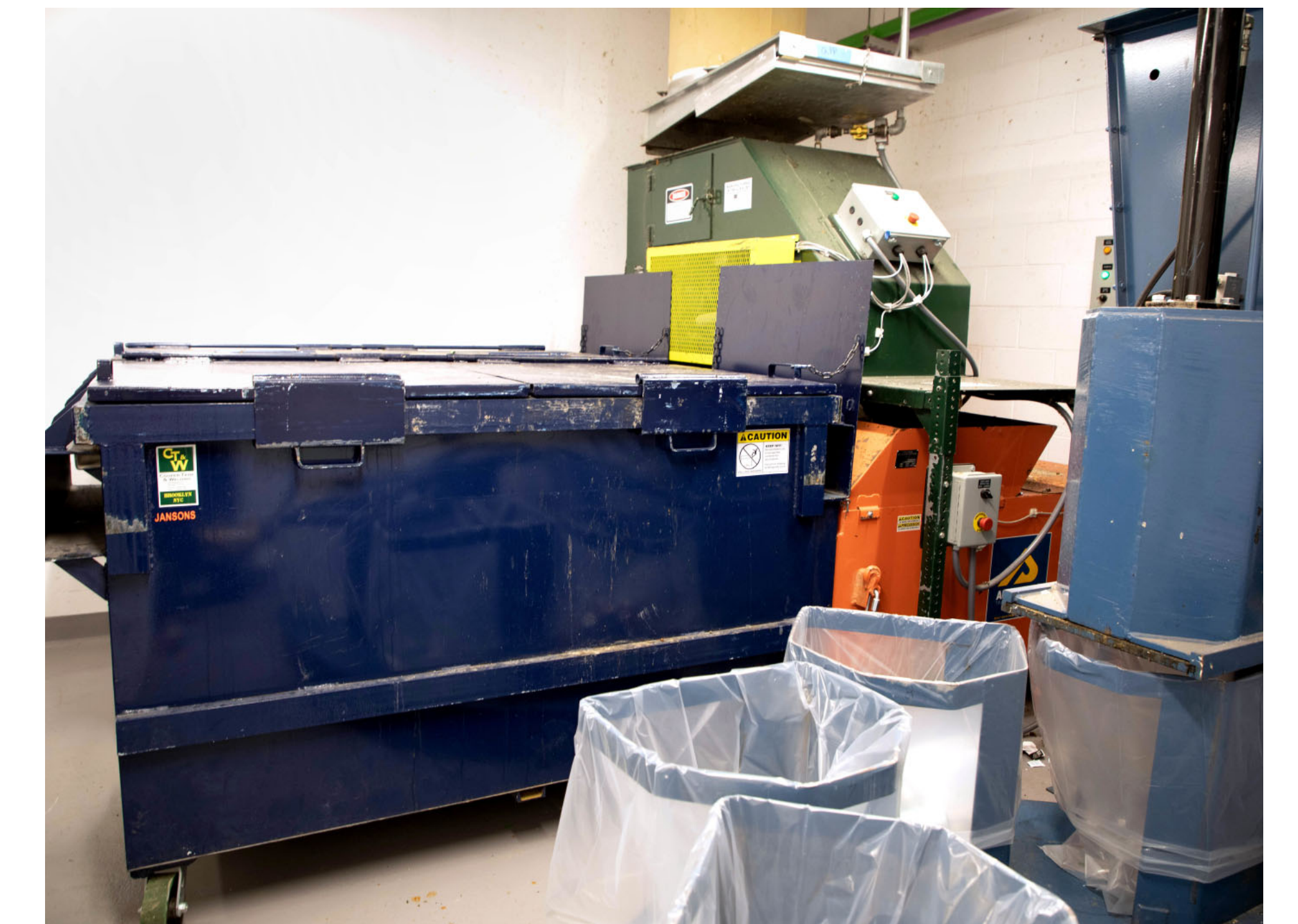
Clockwise from top: refuse room, loading dock exterior, vertical trash compactor, and bag carousel for MGP
